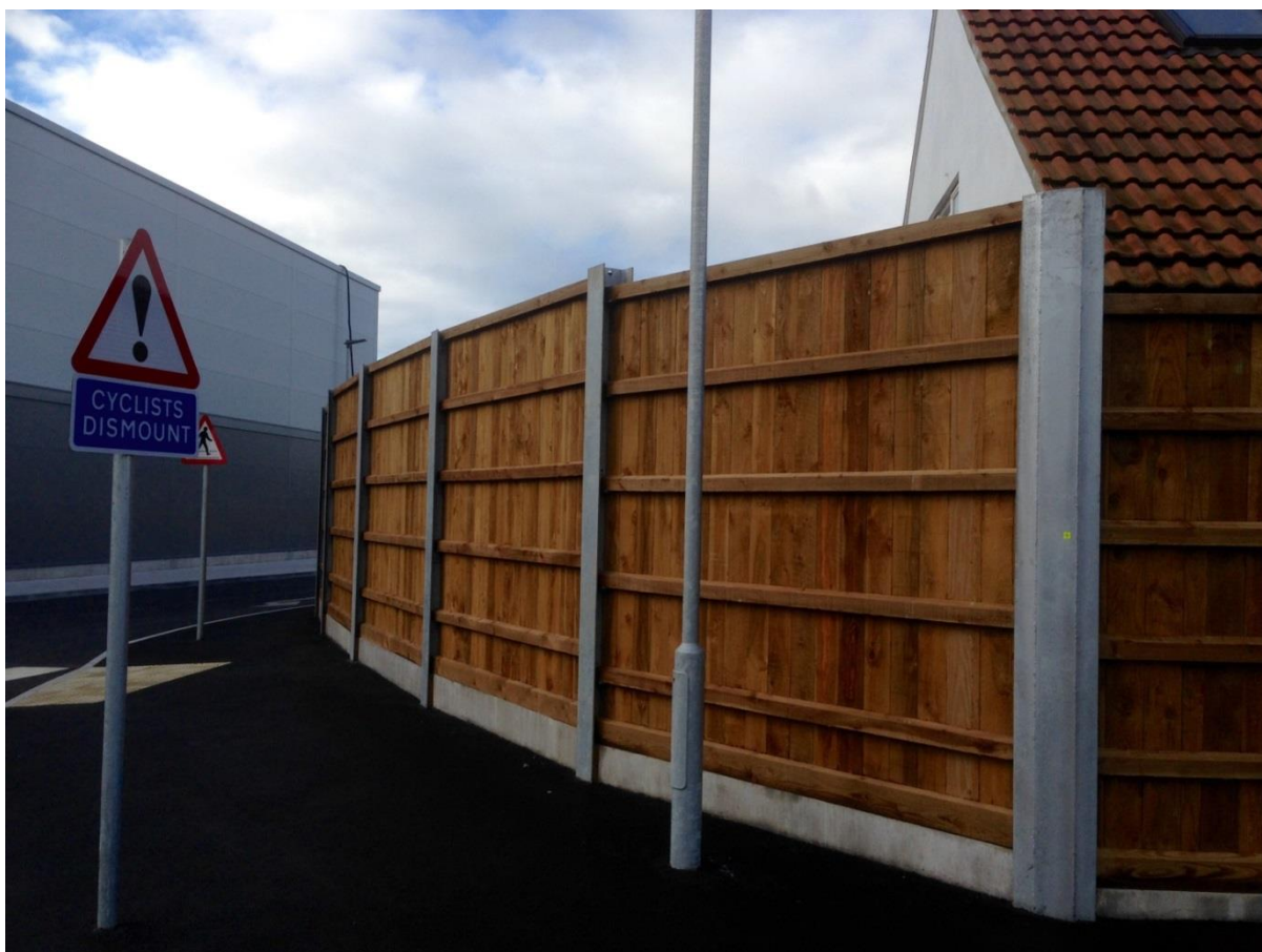
Photograph 4: An example of sound proof fencing.
